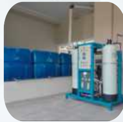
Grade Water Treatment
