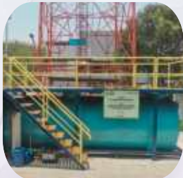
Wastewater Treatment Installation
