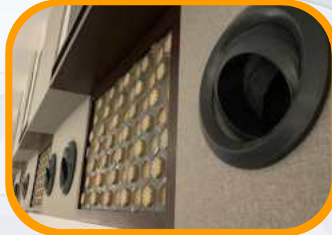
Element 2 Indoor Environmental Quality (HVAC)
