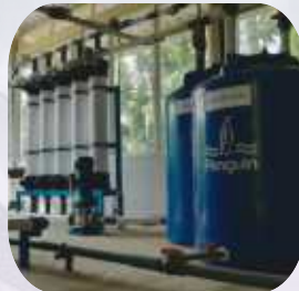
Water Treatment Plant for Student Housing
