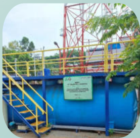
Wastewater Treatment Installation
